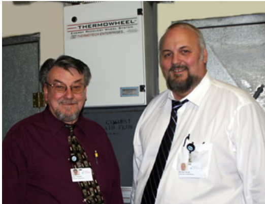
John Roberts and Mike Pascale in front of AHU unit with Thermowheel TR-474 control panel.
